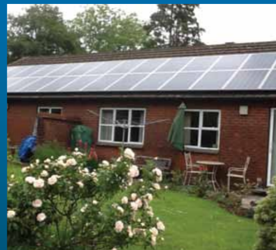
Solar panels at Sutcliffe Close, funded by SDR.
